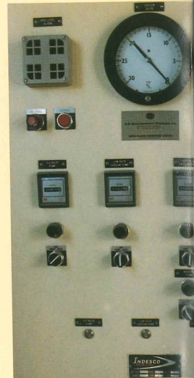
Typical Control Panel
