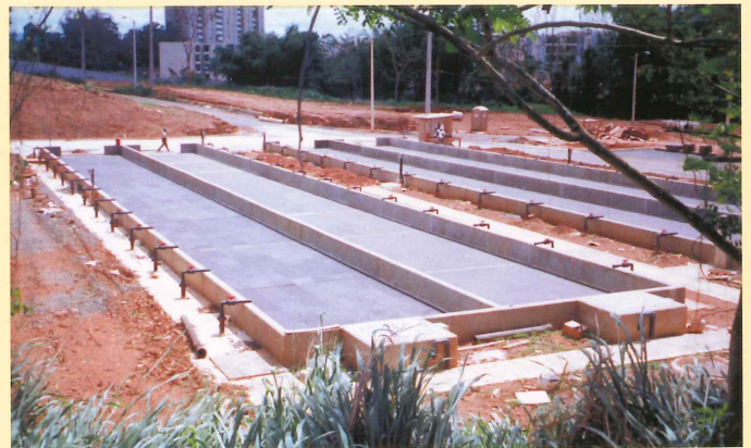
Four Bed VSDB Facility at a 120 MGD Water Treatment Plant in Sergio Cuevas, Puerto Rico.
