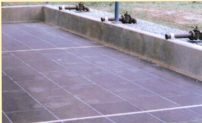
Typical VSDB with Distribution Inlet Lines Shown.
